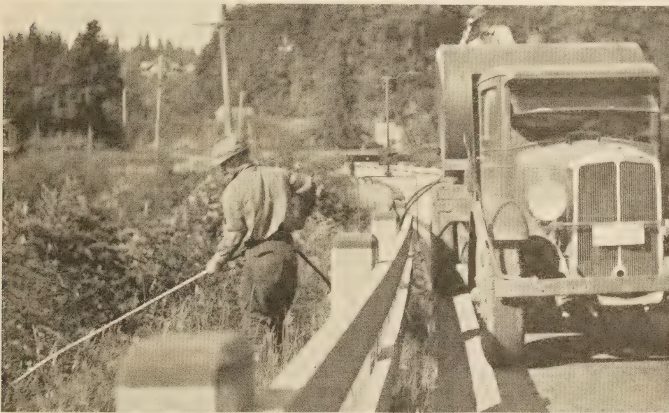
Truck equipped with U-Shaped Device for Spraying Around Posts and Under Rail. Weeds Behind Rail Are Being Sprayed Using a Pipe Attachment.
